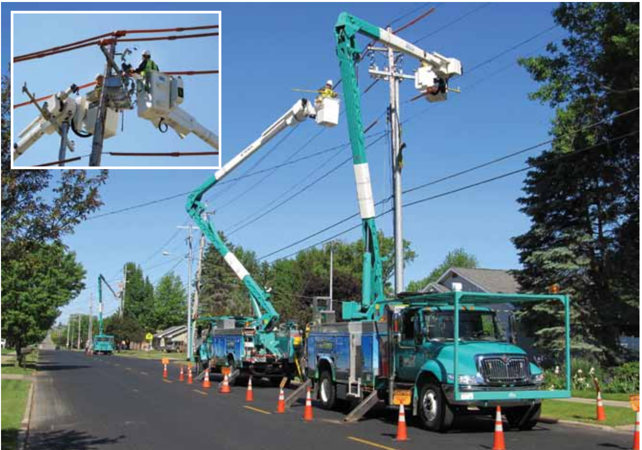
Crews cover energized equipment to allow for new 795 ACSR installation. Linemen use the jib and winch feature to remove an existing capacitor bank (inset).
